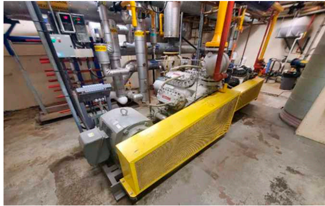
Figure 5: NPA Refrigeration Plant
